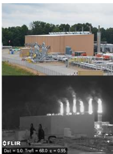
Earthworks - Compressor station emissions containing VOCs made visible with a FLIR Camera
